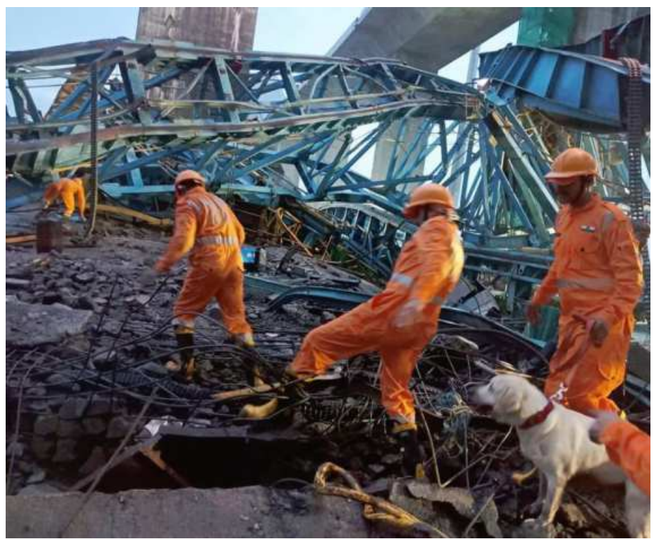
ROAD TO NOWHERE. NDRF personnel carry out a search and rescue operation after a crane fell on a bridge slab on the under-construction Samruddhi Expressway, at Shahapur Tehsil of Thane district, on Tuesday. Twenty people were killed and three others were injured in the accident. PH
